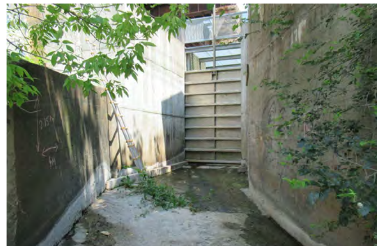
4a) The sluiceway is a concrete channel with a metal gate to carry excess water.
