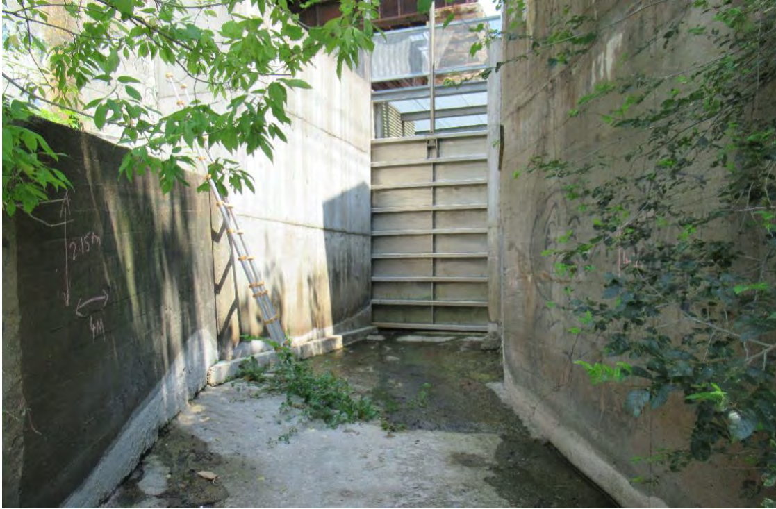
Exhibit 5-1: The sluiceway is a concrete channel with a metal gate to carry excess water.
