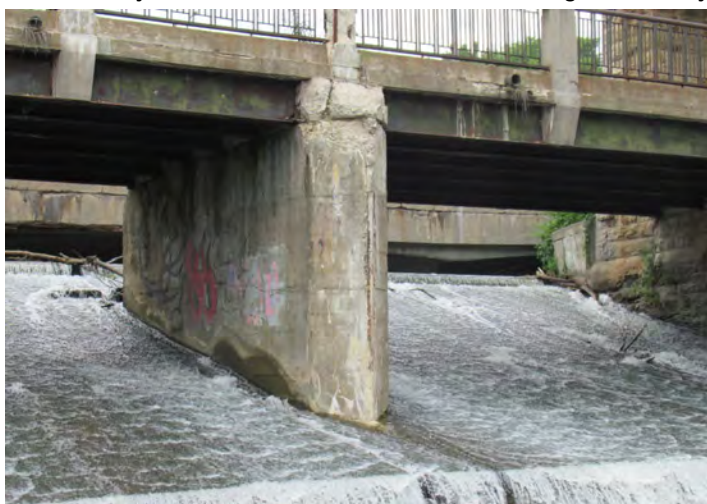
Exhibit 5-2 The spillway forms a weir to control the Speed River elevation, previously used for the now-removed Allan's Mill
