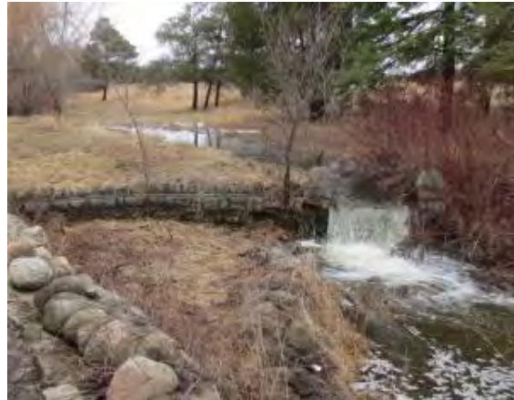
Image 26: Clythe Creek, fieldstone weir with cut stone terrace wall (City of Guelph Heritage Planning)
