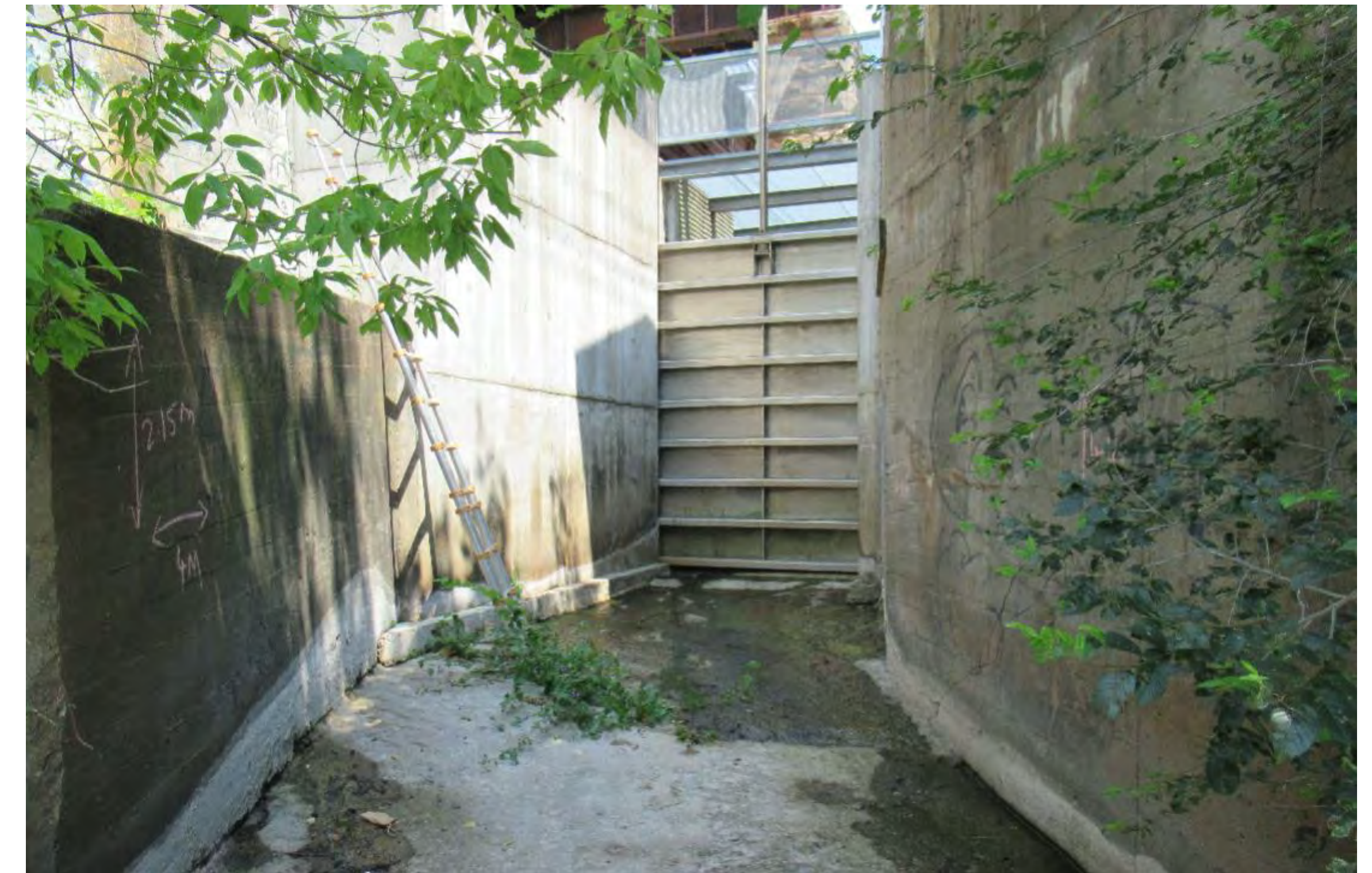
23a) The sluiceway is a concrete channel with a metal gate to carry excess water.
