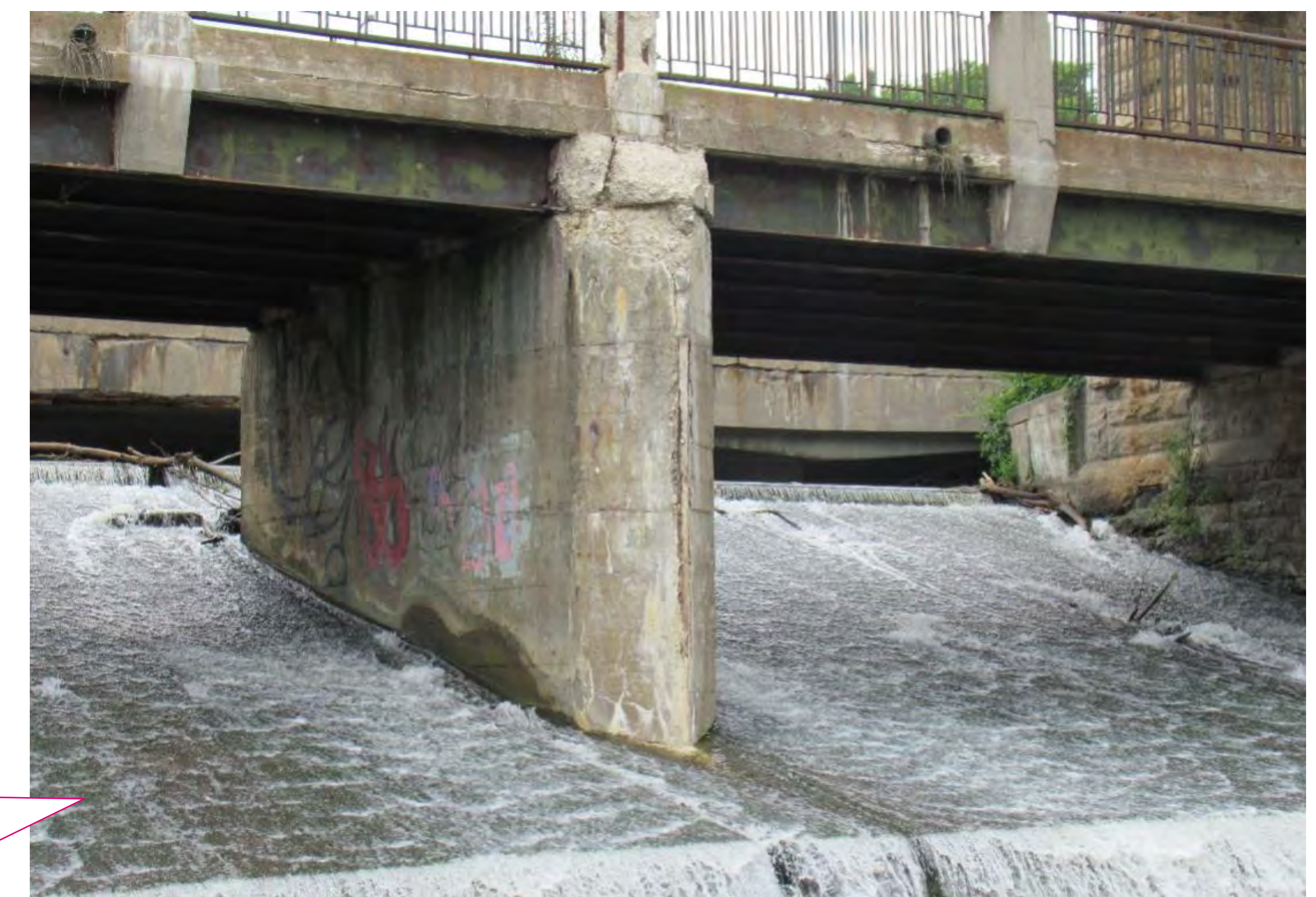
23b) The spillway forms a weir to control the Speed River elevation, previously used to for the now-removed Allan's Mill.
