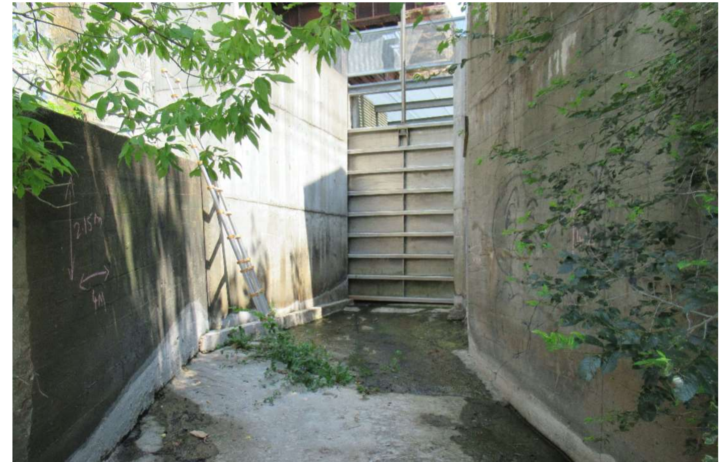
4a) The sluiceway is a concrete channel with a metal gate to carry excess water.
