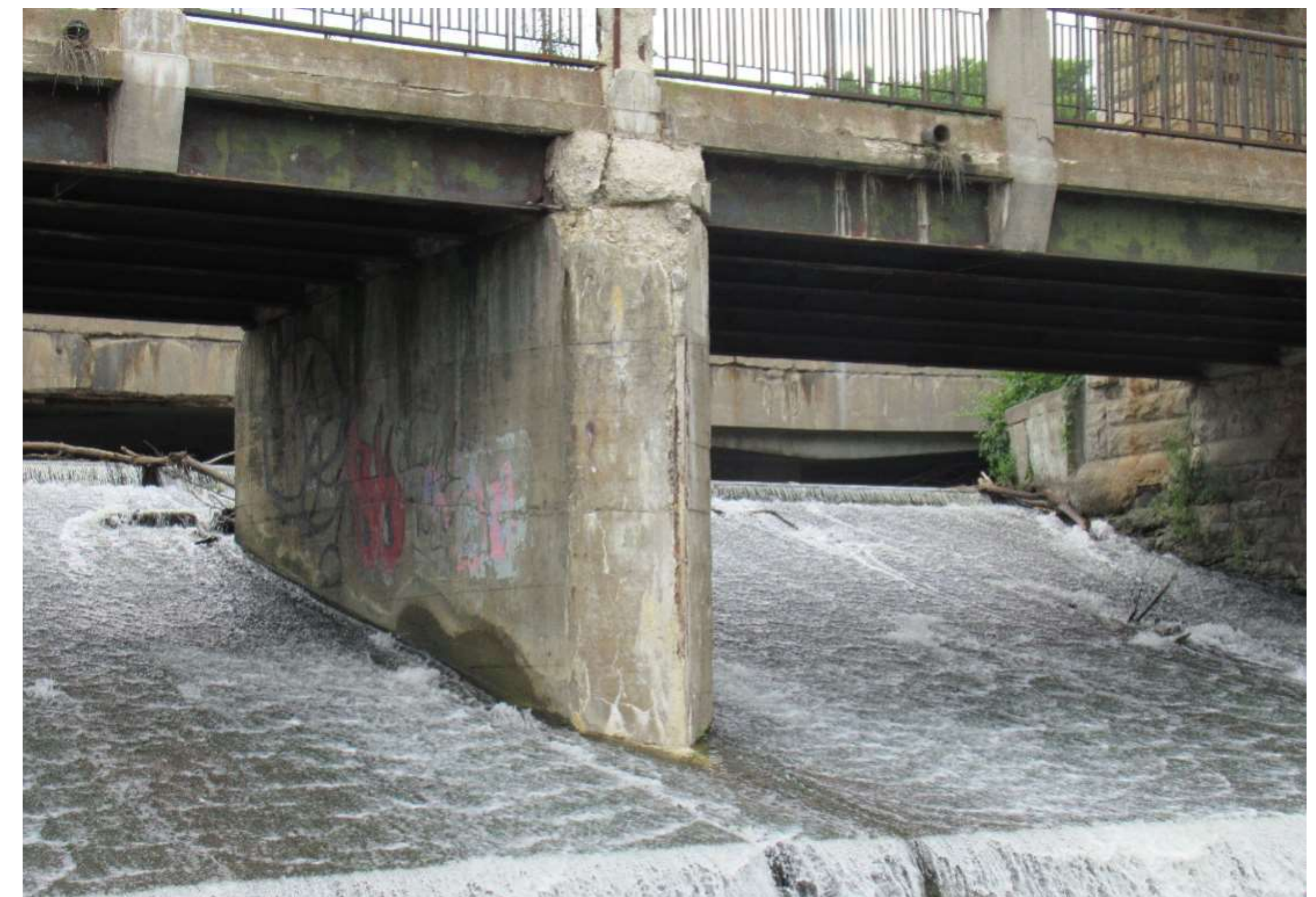
4b) The spillway forms a weir to control the Speed River elevation, previously used for the now-removed Allan's Mill.
