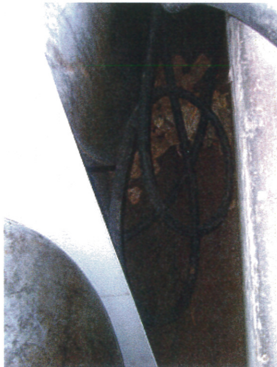
Photograph 6: A view of the bottom of the concrete enclosure for the ASTs.
