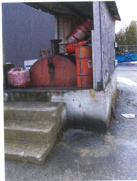
Photograph 8: A view of the staining on the concrete enclosure and asphalt.
