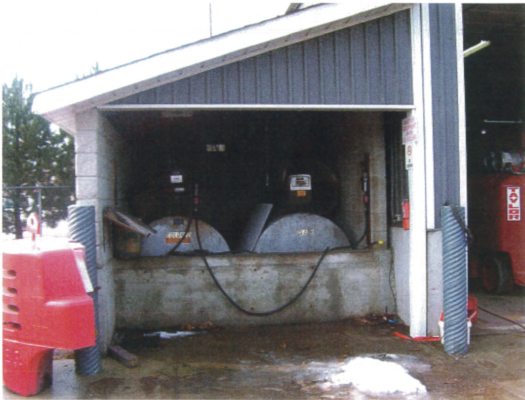
Photograph 5: A view of the diesel ASTs on the south side of the building.
