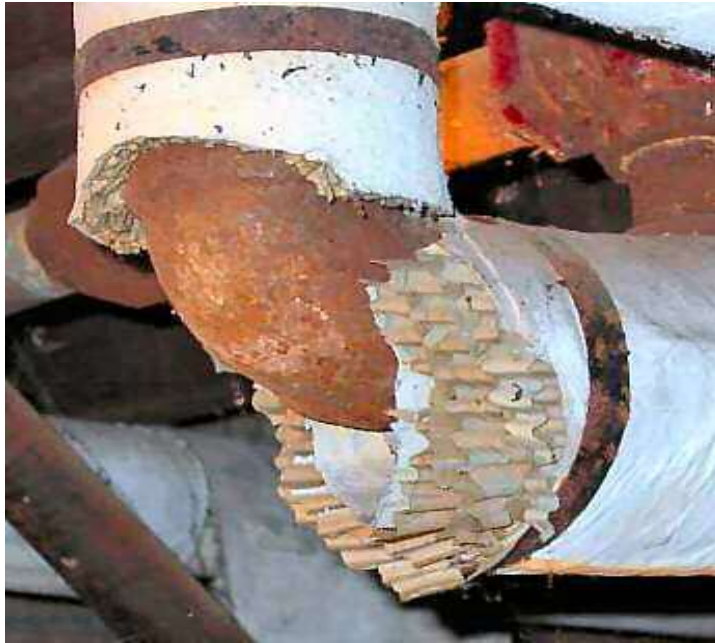
Damaged Asbestos Pipe Elbow
