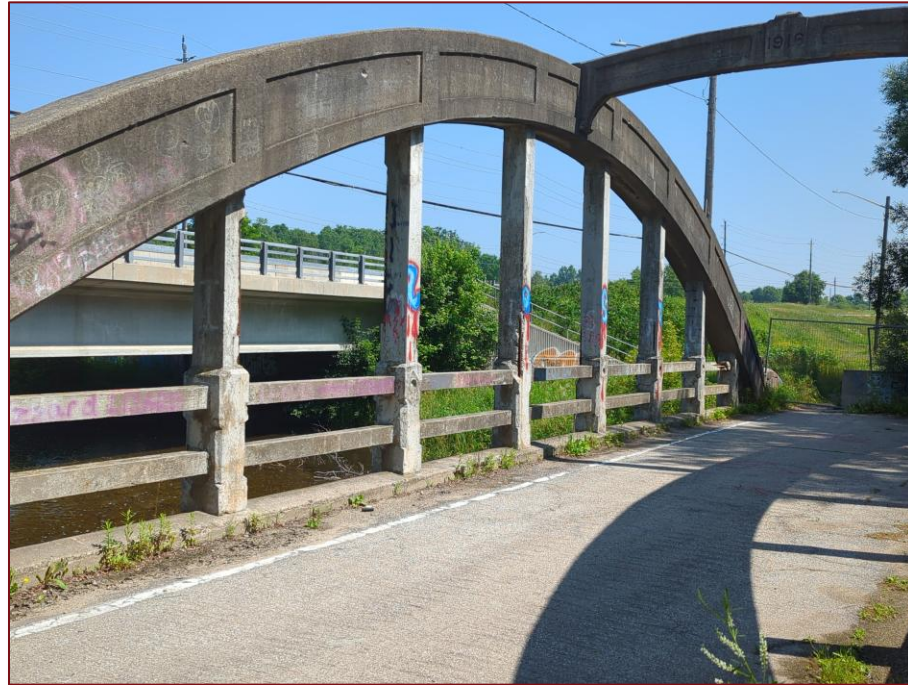
Image 14: Exposed Reinforcement Bars of Hangers
