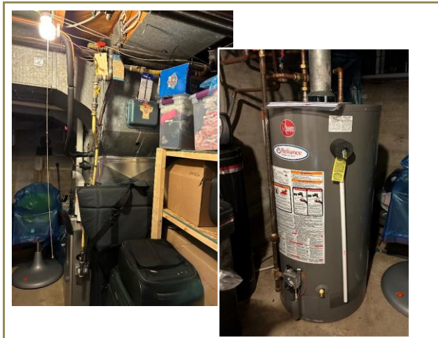
Photograph 9: Hot water boiler and natural gas forced air furnace in basement of the building.
