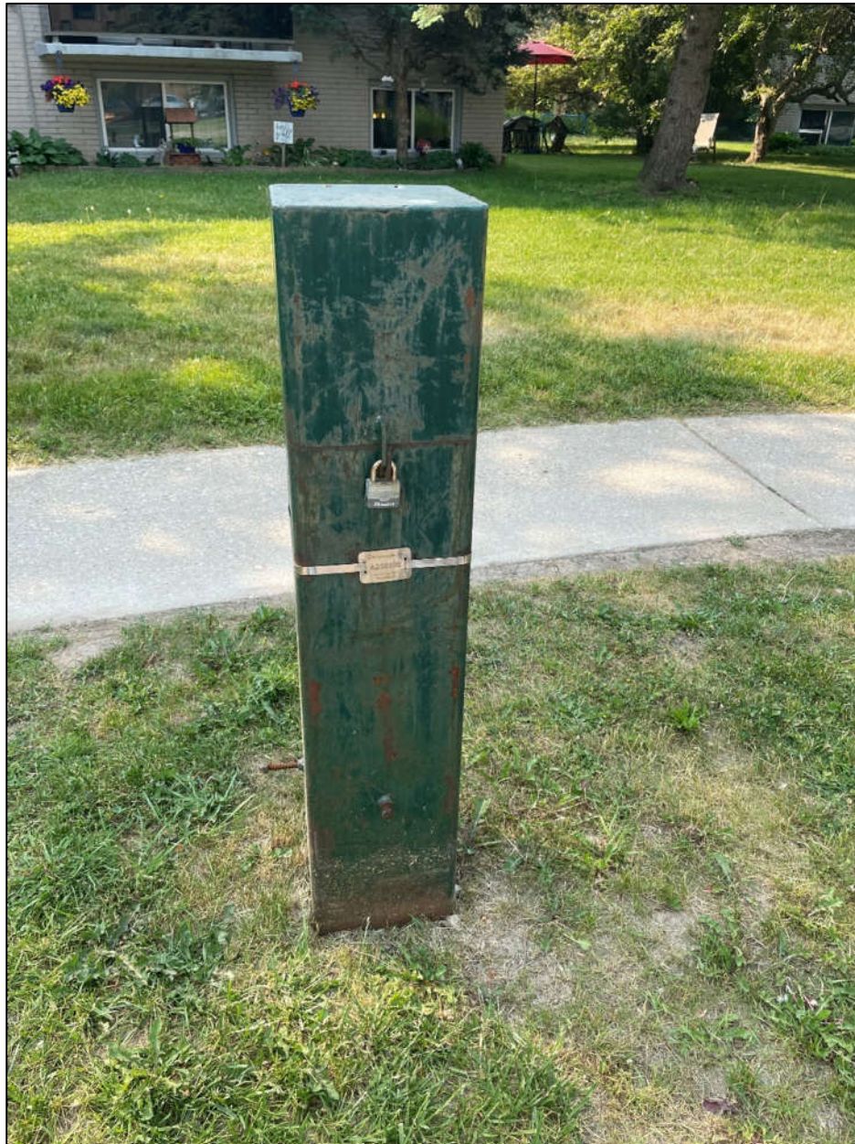
Figure 40 View of a monitoring well located on the south edge of Manhattan Court southeast of the Site, facing south.
