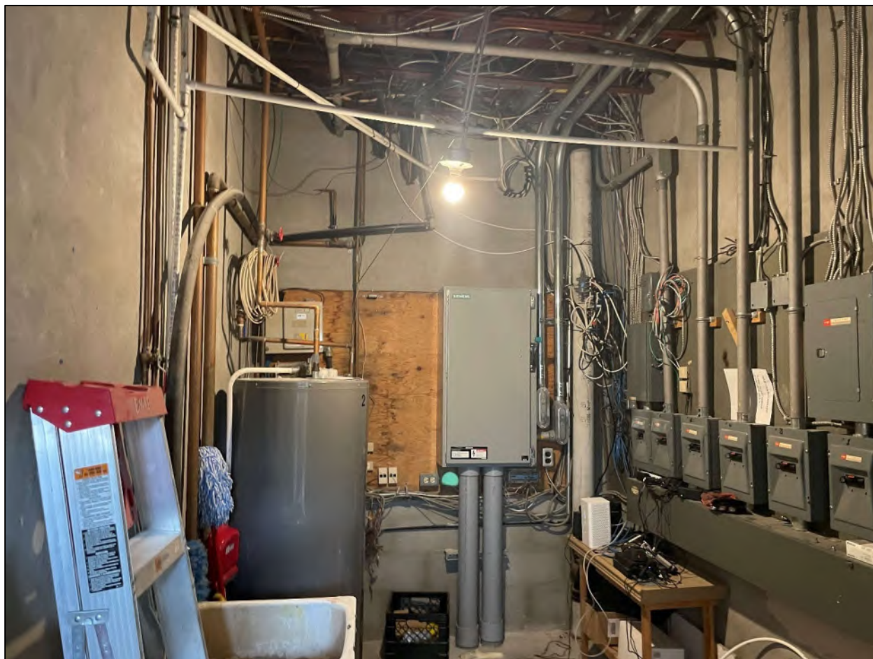
Figure 23 View of the mechanical room in the basement of 317 Speedvale Avenue East.
