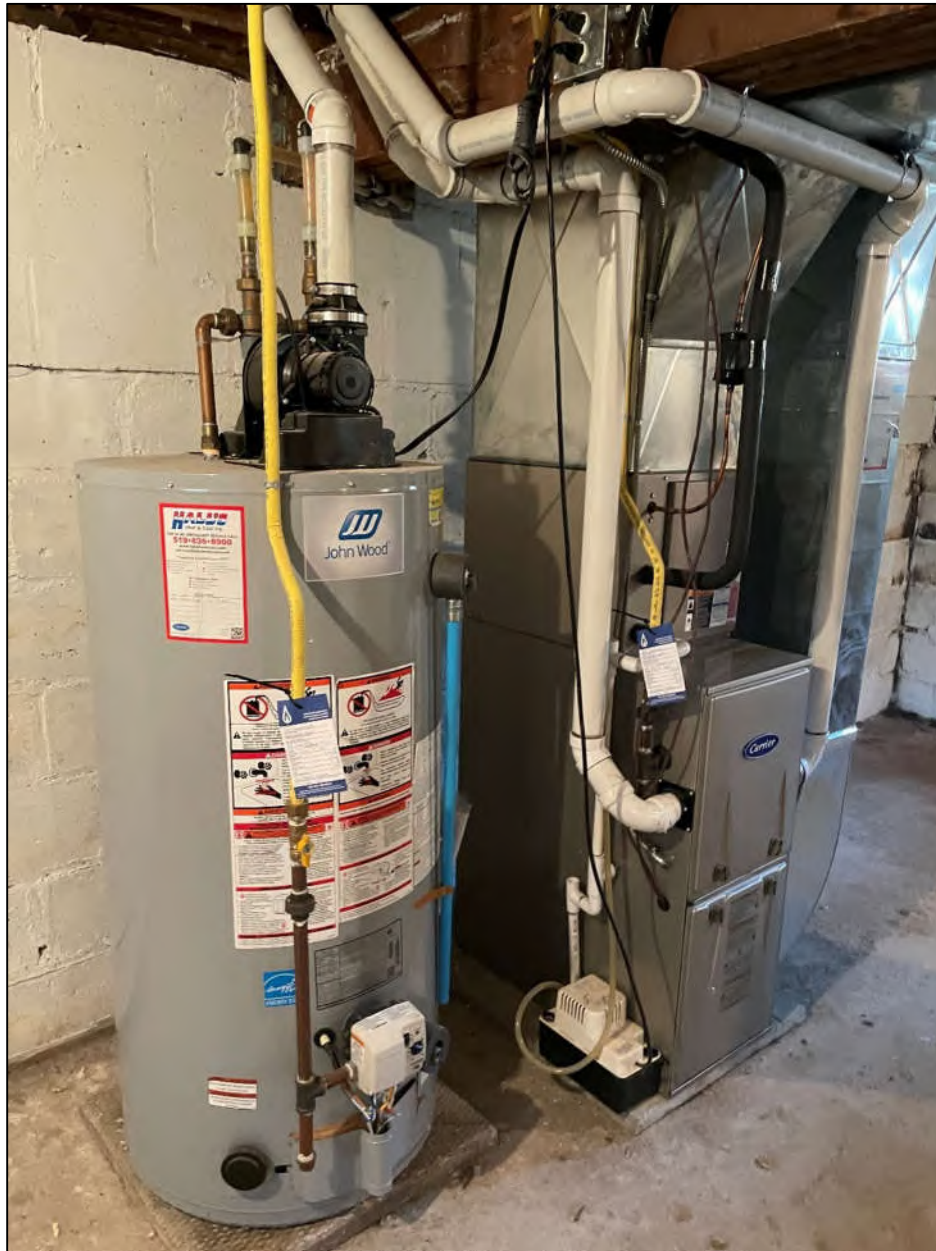
Figure 15 View of the furnace and water heater on the southeast wall of the basement in 309 Speedvale Avenue East, facing southeast.
