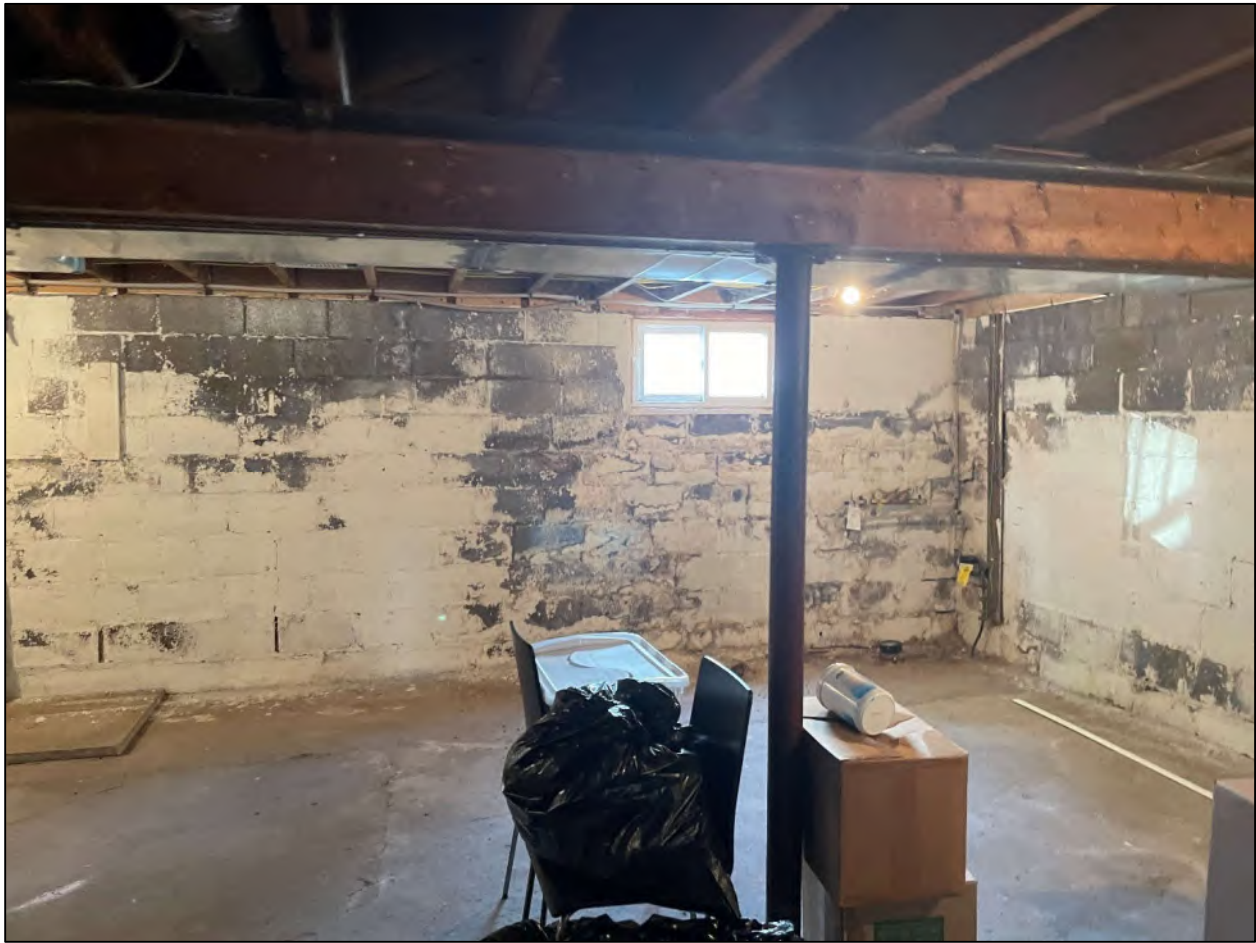
Figure 13 View of the southwest wall of the basement in 309 Speedvale Avenue East, facing southwest.
