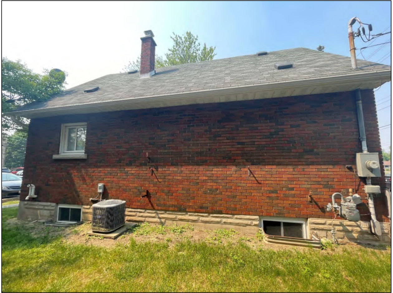
Figure 5 View of northeast elevation of 309 Speedvale Avenue East, showing natural gas service and AC unit on northeast wall, facing southwest.
