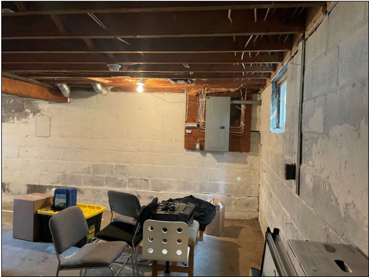
Figure 12 View of the electrical panel in the northern corner of the basement in 309 Speedvale Avenue East, facing northwest.
