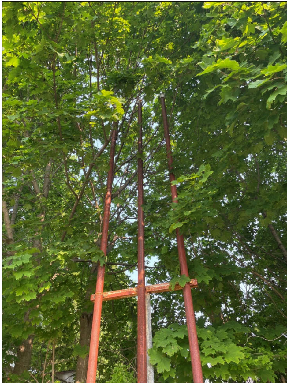
Figure 35 View of vents indicating historical underground storage tanks on the northwest property boundary of the vacant lot located on the west corner of Speedvale Avenue East and Stevenson Street North (324 Speedvale Avenue East), facing west.
