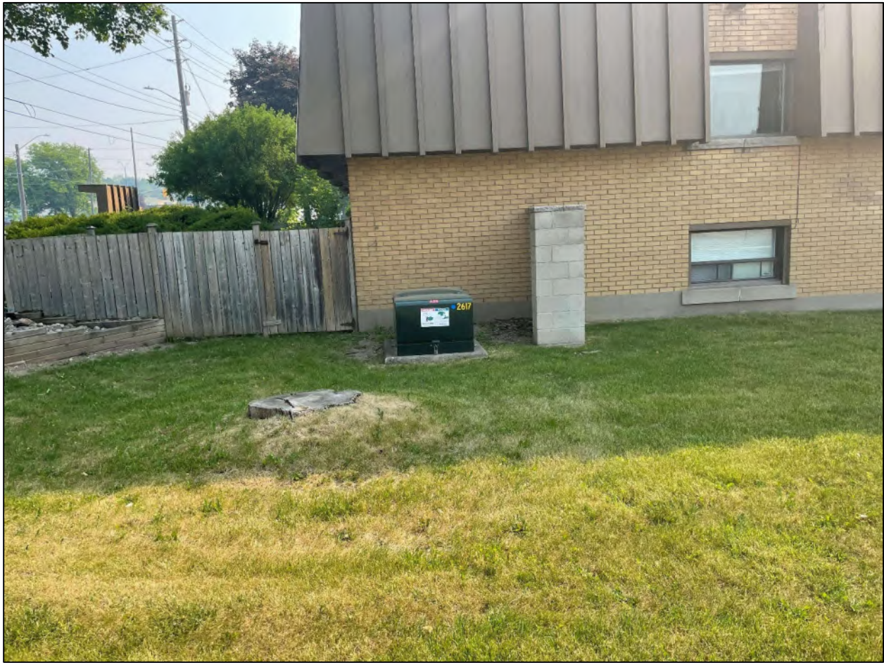
Figure 37 View of a pad mounted transformer on the southwest side of the neighbouring dentist office to the northeast Site boundary, across Manhattan Court, facing northeast.
