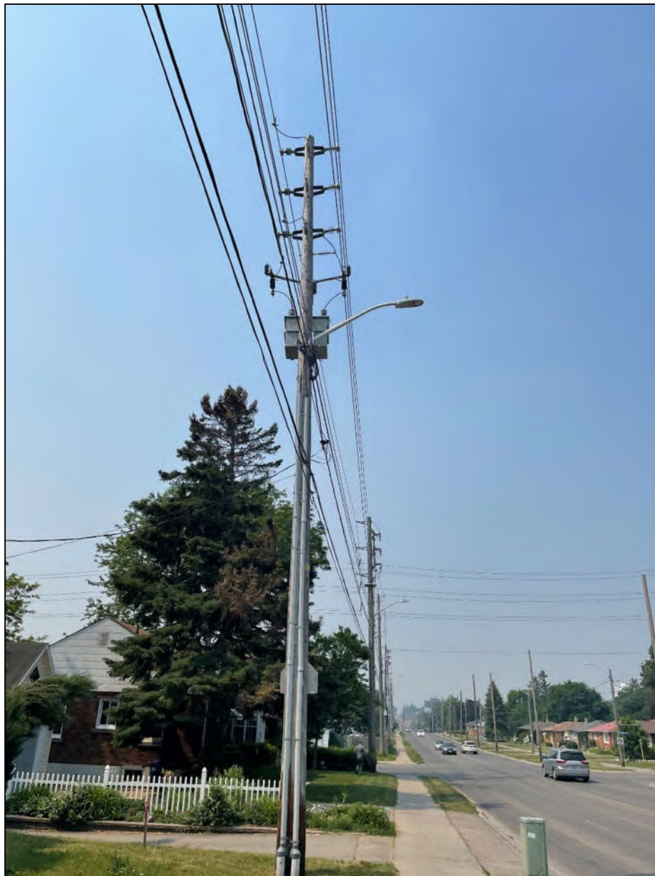
Figure 3 View of Speedvale Avenue East and a pole mounted transformer in front of 303 Speedvale Avenue East, facing southwest.
