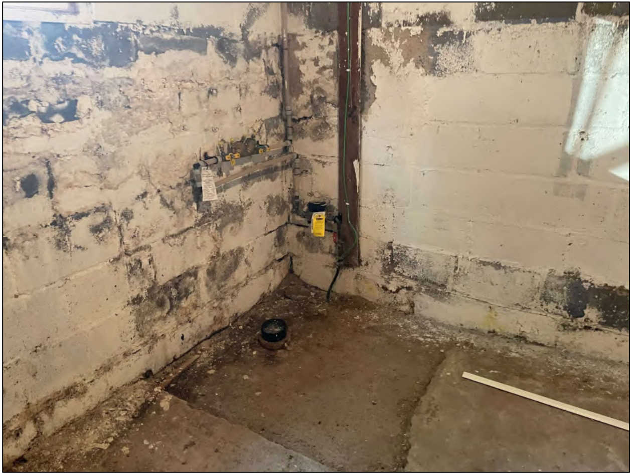
Figure 14 View of the west corner of the basement in 309 Speedvale Avenue East showing sump location, facing west.
