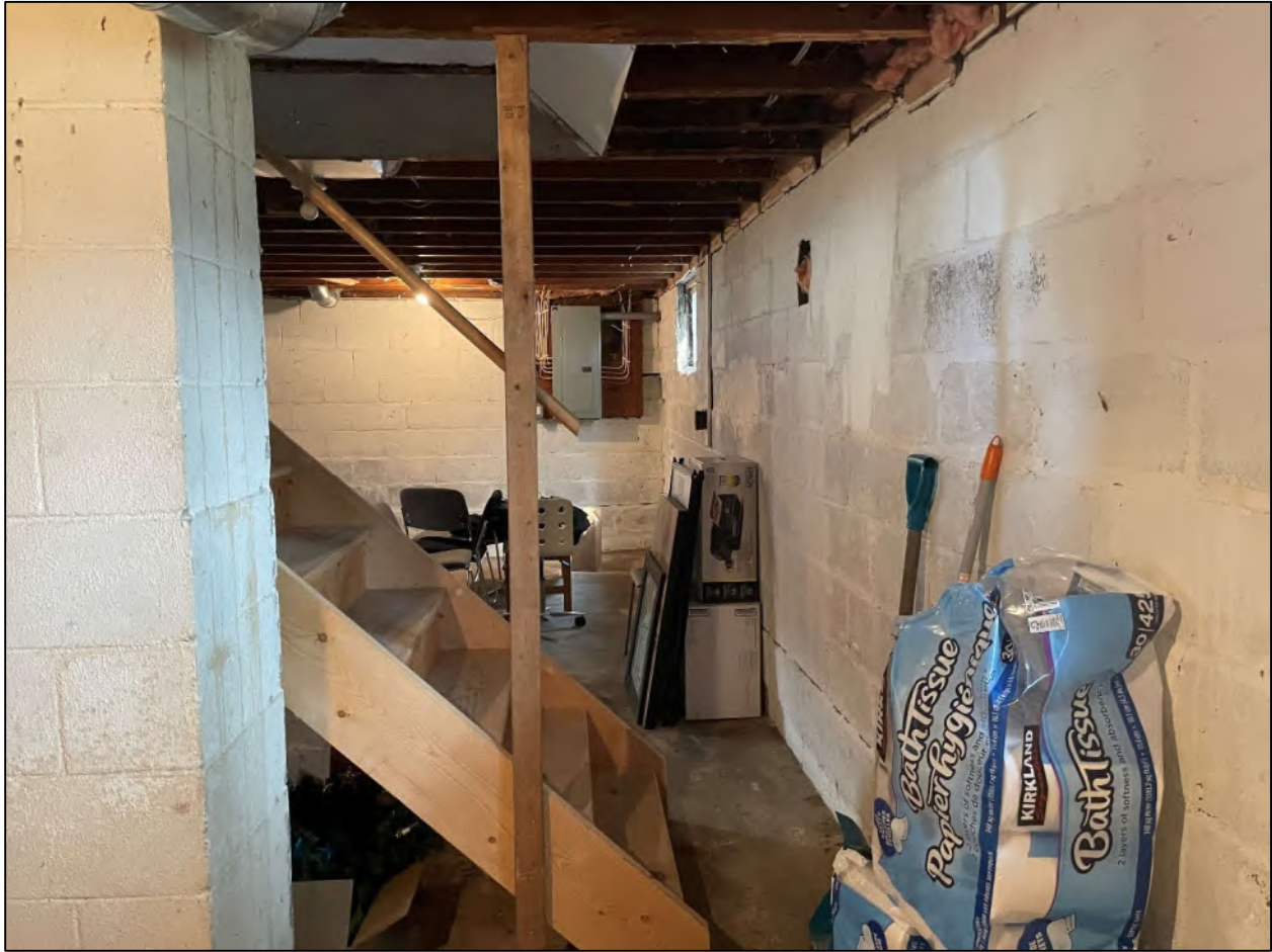
Figure 11 View of stairs in the basement of 309 Speedvale Avenue East, facing northwest.
