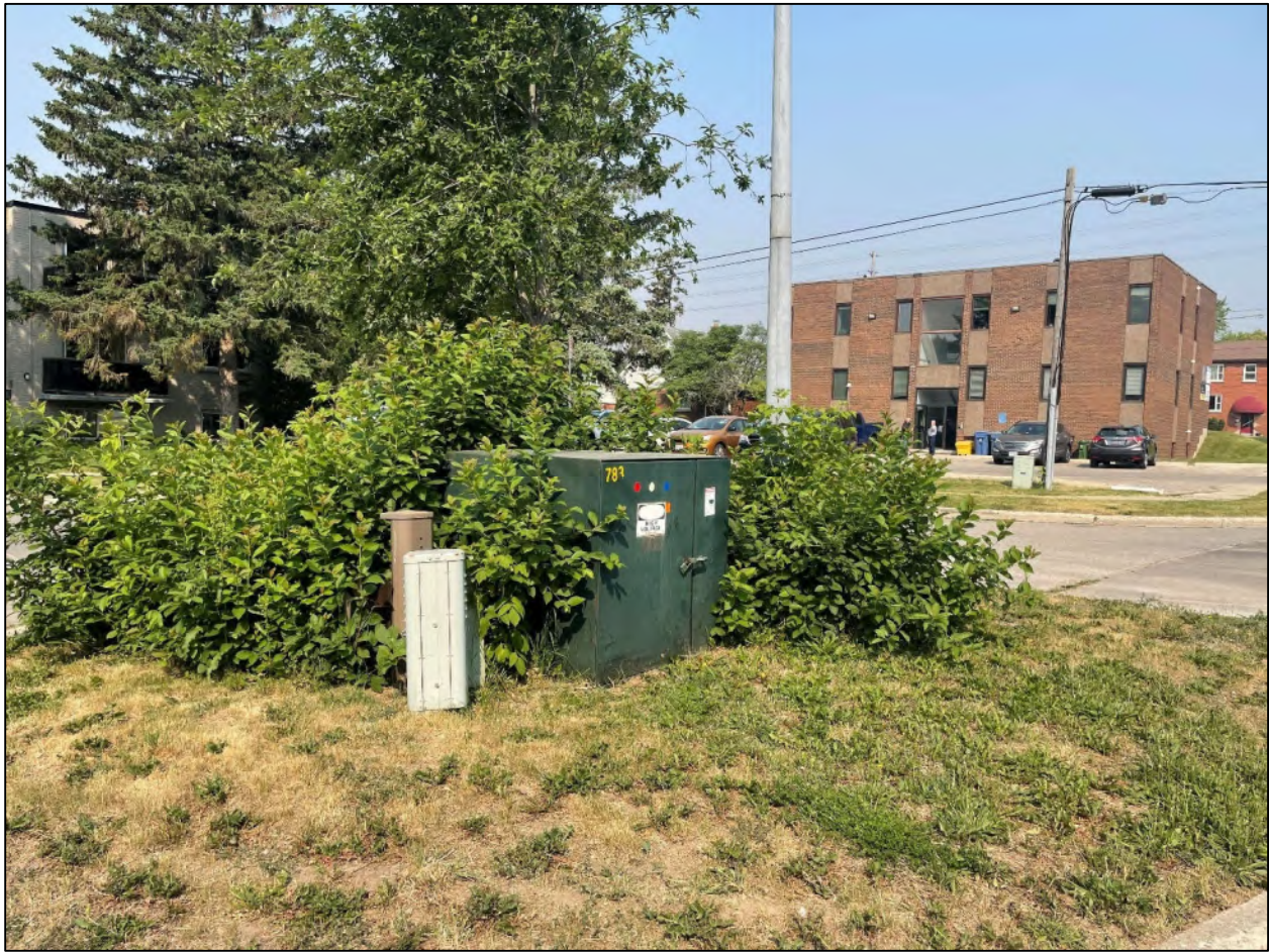
Figure 39 View of a communications box and a pad mounted transformer located in the center of Manhattan Court adjacent to the east Site boundary, facing west.
