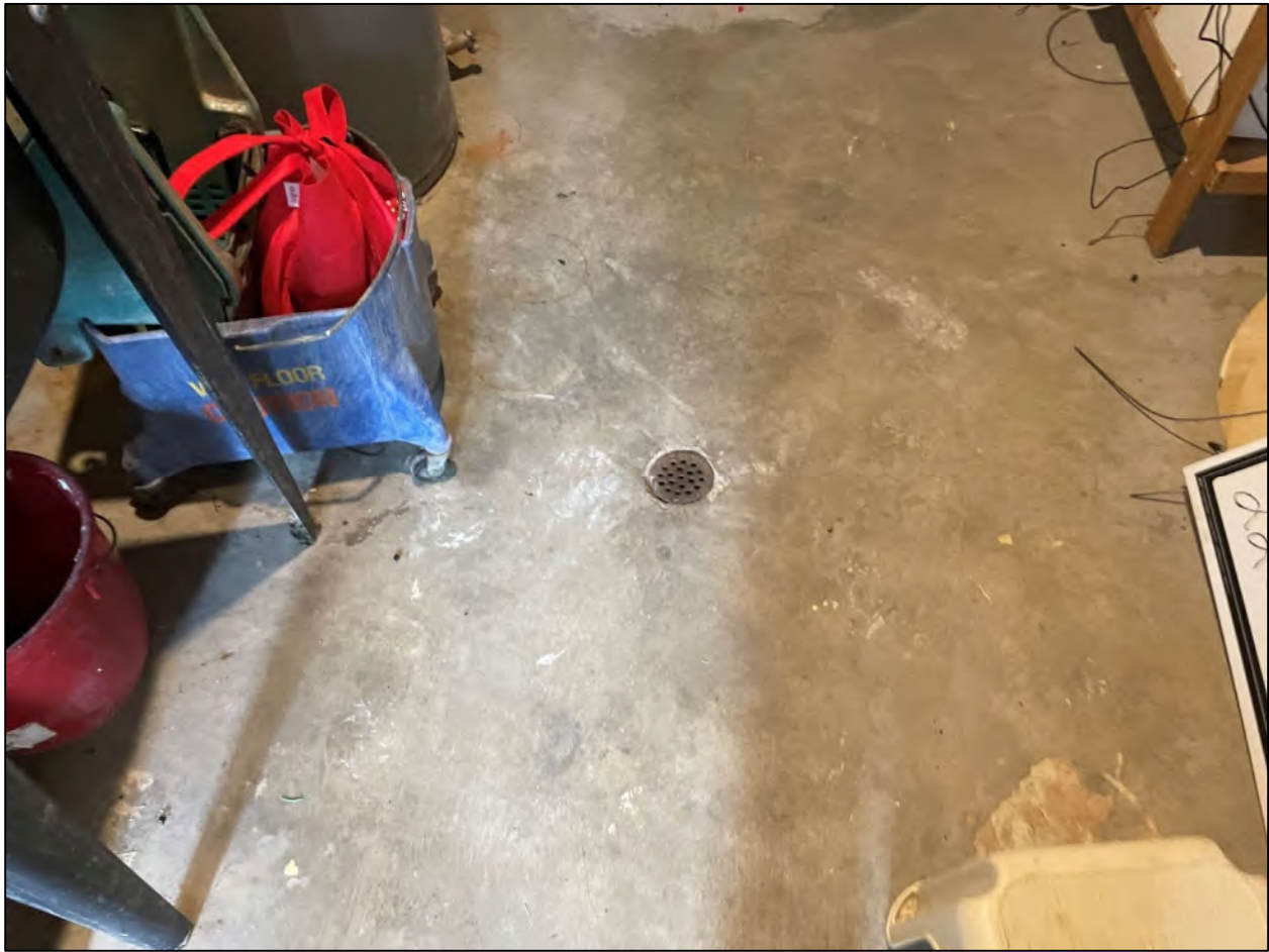
Figure 24 View of a floor drain in the center of the mechanical room in the basement of 317 Speedvale Avenue East.
