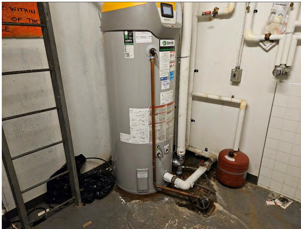
Photo 8: Hot water heater located on second floor of Galaxy Cinemas. Leaking water observed on floor at base of water heater.
