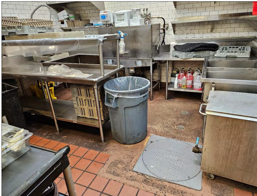
Photo 26: Kitchen area of State & Main. Grease trap observed on floor.
