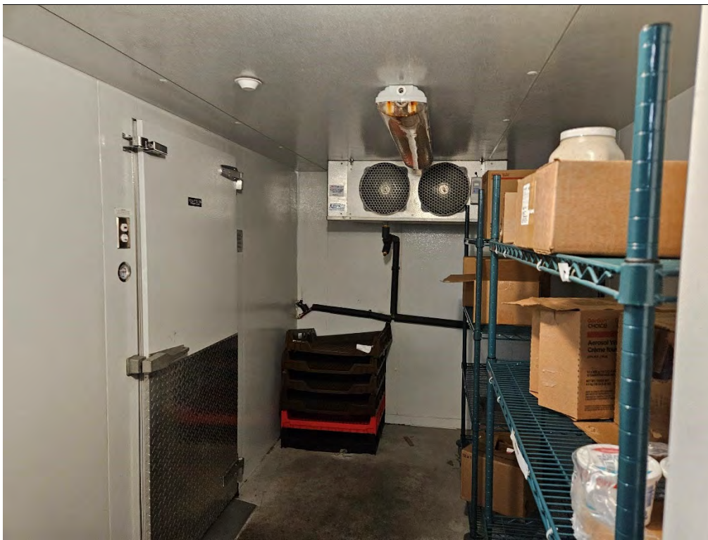
Photo 6: Refrigeration units located in Galaxy Cinemas.
