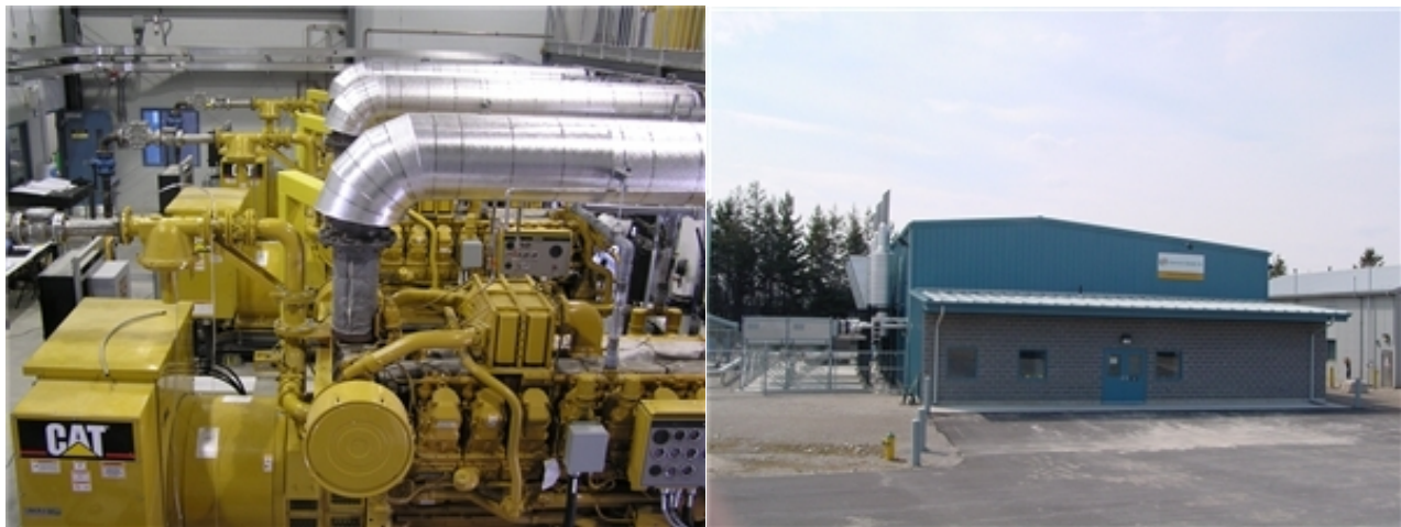
Figure 19: Eastview Landfill Gas Energy Plant Photos [7]
