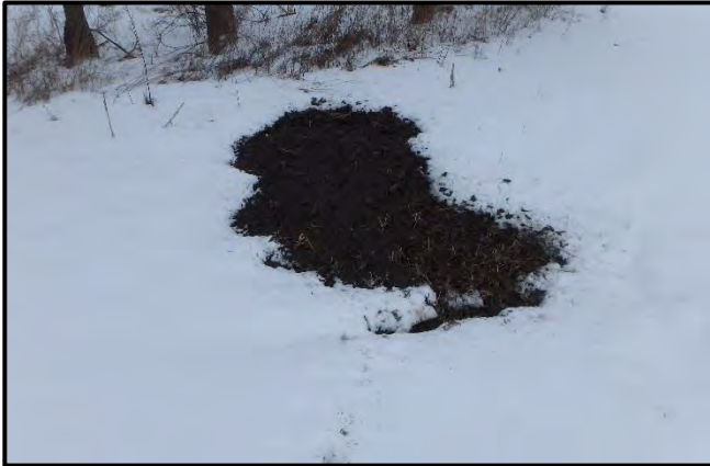
Photo 15. Seep at 2162 Gordon Street (March 17, 2017)
