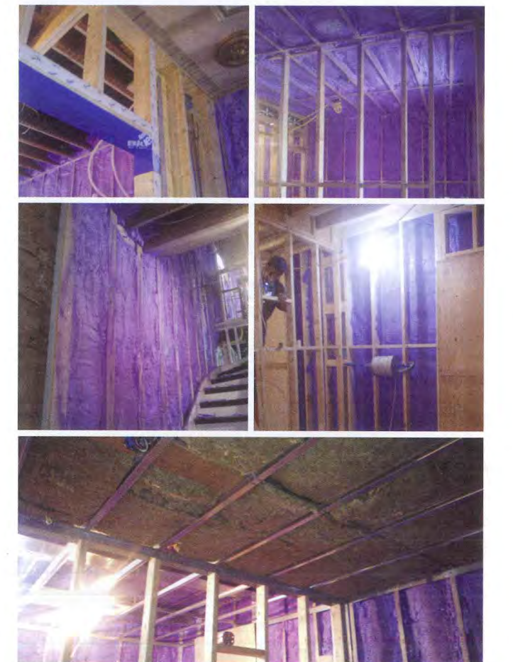
Urethane foam insulation was applied inboard of the exterior masonry walls. The spray foam was coupled with a unique vented drying airspace that helps the double-wythe historic masonry dry on both the inboard and exterior faces after insulation.
