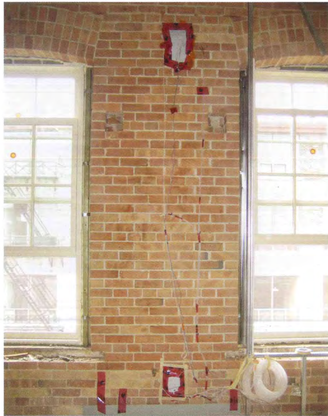
Figure 3: Monitoring equipment at the top and bottom of the vented airspace cavity (prior to application of the polymer mesh system).
