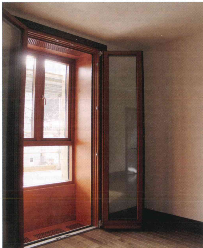
South-facing windows were doubled up as core and perimeter windows were separated by a 150 mm vertical plenum for gathering solar heat.
