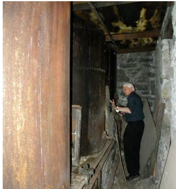
14. Building #1, storage tanks (Source: City of Guelph)
