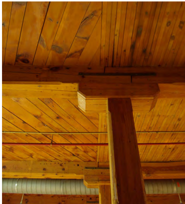
42. Building #2d, heavy timber structure and wood ceiling. (Source: City of Guelph)
