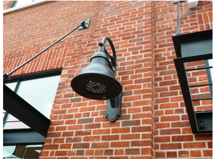
Pedestrian scale lighting featured attached to a building wall.
