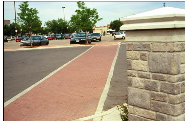
The above photograph shows a close up view of the extension of the walkway into the retail plaza, which was discussed above.
