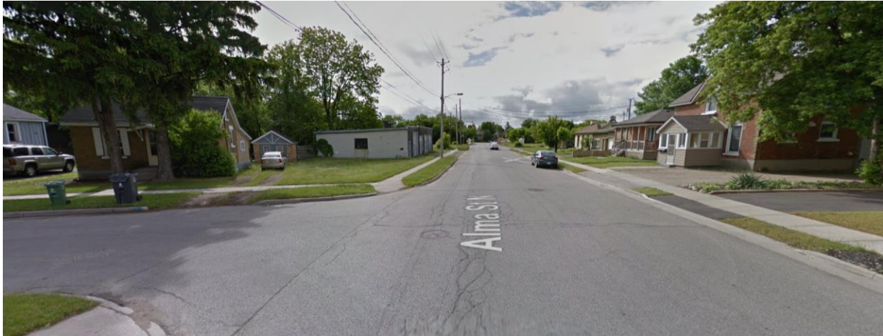
Figure 38. Example of Road Segment in Fair Category (PCI 40 to 59)
