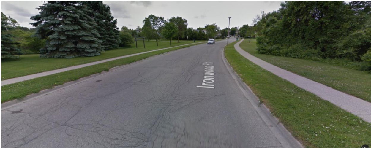
Figure 39. Example of Road Segment in Poor Category (PCI 20 to 39)
