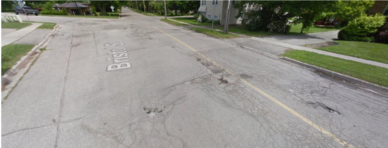
Figure 40. Example of Road Segment in Very Poor (PCI <20)
