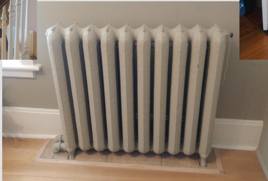
Original radiators, 2018 (City of Guelph)
