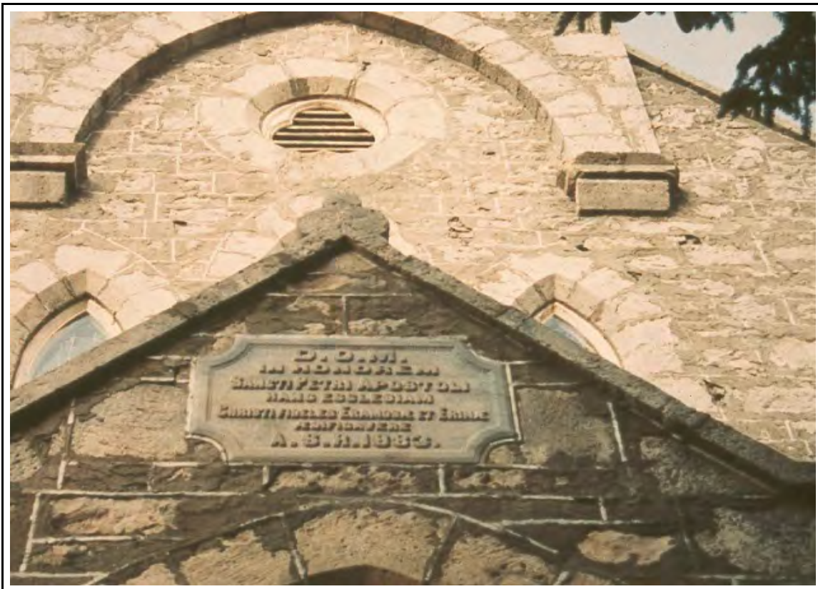
Photo. 8: Further deterioration is evident after 20 years
