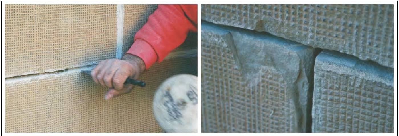
Photos.18 & 19: Cutting out over-loaded face bedded stone mortar joints using hand chisels (left) caused damage to the masonry which was not created when grinders were used. This was due to unusually high loads imposed on the outer wythe of masonry following roof reconstruction work carried out 30-years previously.
