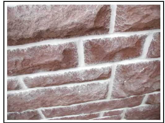
Photos.26. The result of repointing while the face of the masonry is wet.
