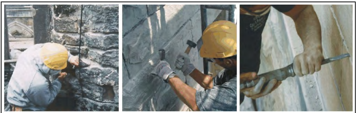
Photo.20, 21 & 22: Removing deteriorated mortar with chisel (left) rake (middle) and lightweight stone carving tool (right).
