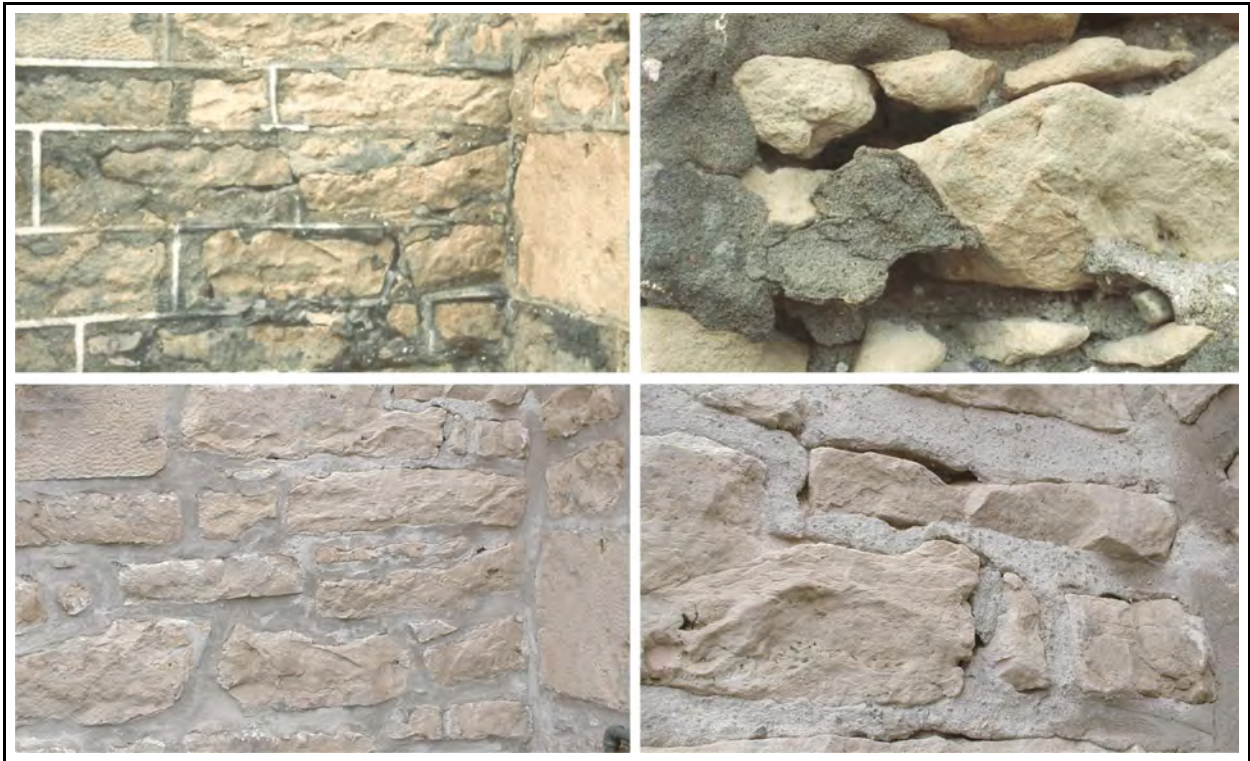
Photo.9 through 12.(Upper Left) Natural stone masonry that has been repointed many times - incorrectly, and (Upper Right) a close up view of accelerated deterioration caused by the incorrect repointing techniques - note the damage caused to the natural stone. (Lower Left) The same area of masonry some 10-years after restoration, and (Lower Right) the omission of inner core rubble grouting has resulted in further deterioration.
