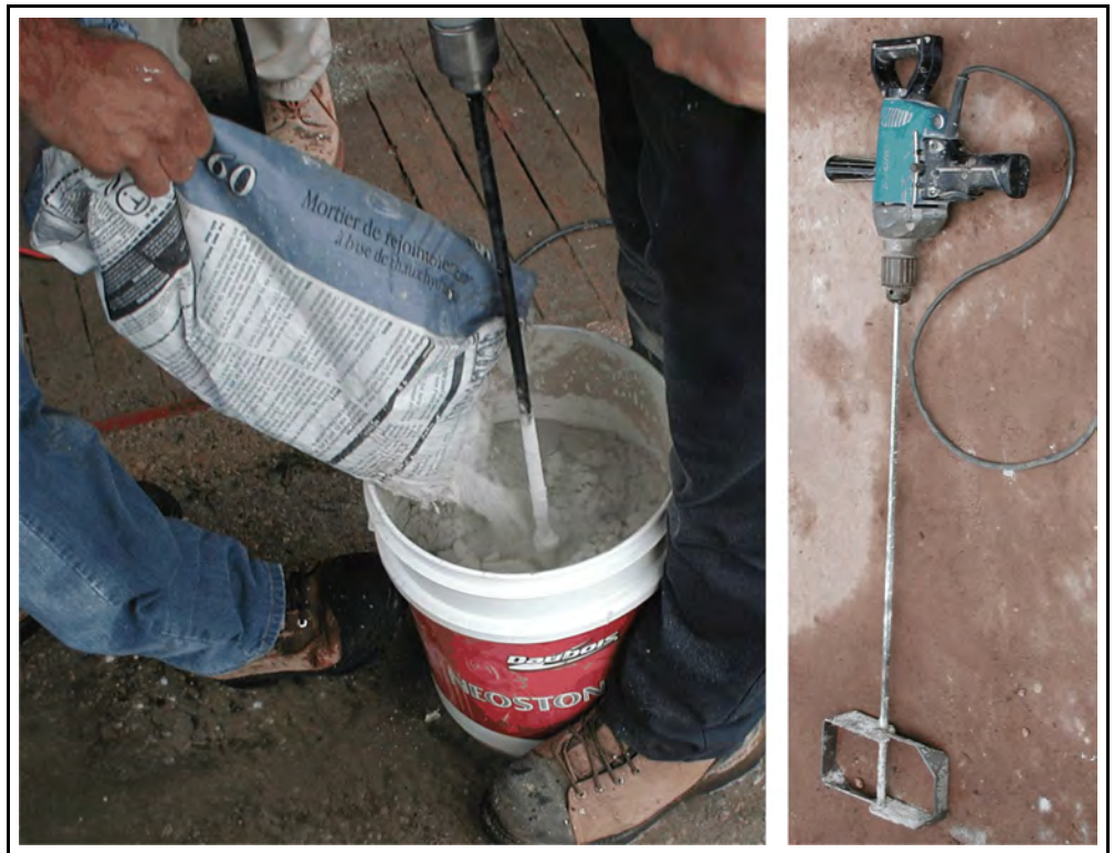
Photos.27 & 28 (Left) Mixing a prepackaged repointing mortar. (Right) A drill and inserted mixing head.
