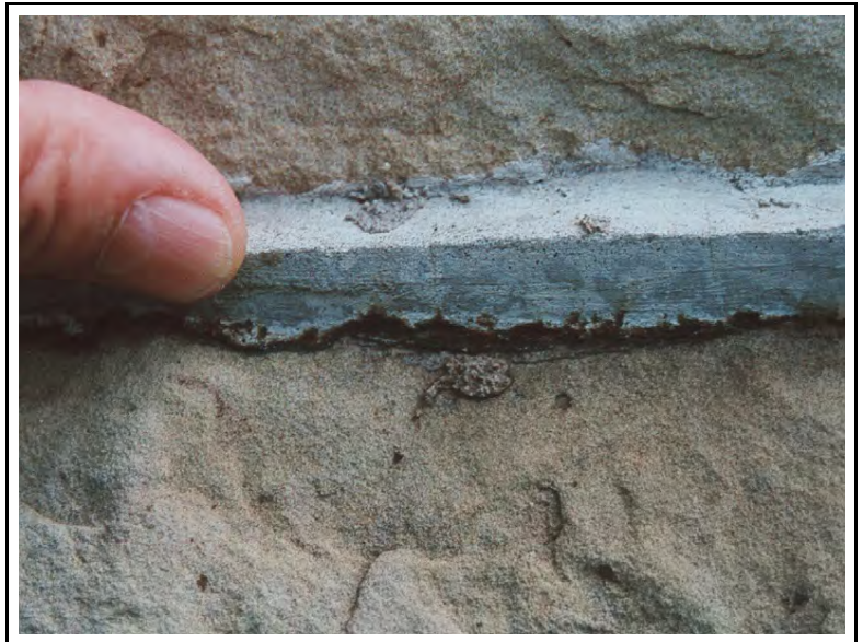
Photo. 1. This hard cement based repointing mortar was applied without cutting out the old mortar and is now causing deterioration to the stone masonry units.
