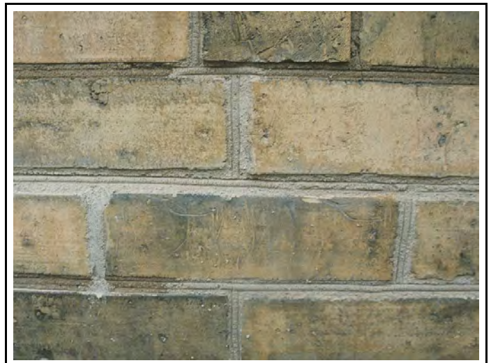
Photo. 6. The repointing of this 100-year old brick masonry attempts to match the original pointing style.
