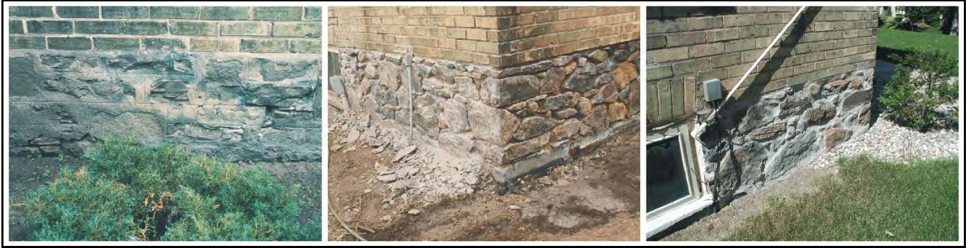
Photos. 13 through 15: A badly repointed foundation wall before, during and after restoration.
