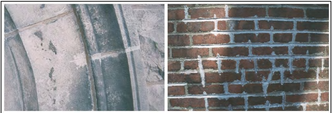
Photos.16 & 17: Damage caused by use of a grinder to remove previous mortar.
